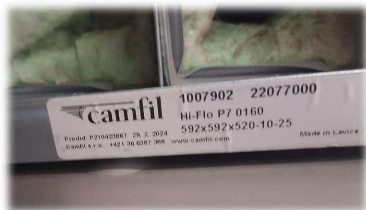
Figure 12: Photo from supply filter
